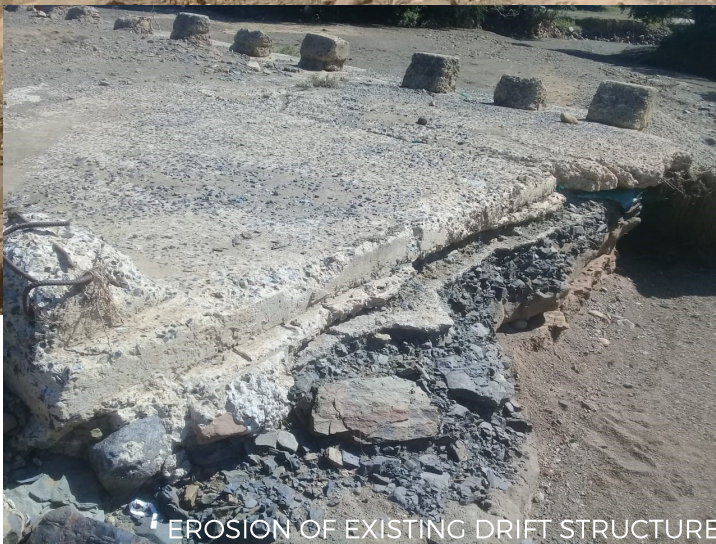
INSPECTION OF FAILED STRUCTURE ON L311
